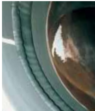
◀ Inside view of the duct with a specially prepared FKM elastomer expansion joint, in the Bielefeld incinerator plant, Germany
