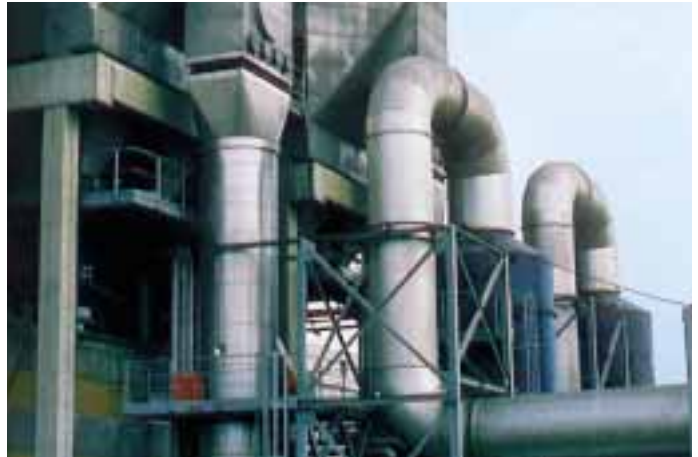
▲ Incinerator plant with flue gas cleaning in Ingolstadt, Germany Medium: flue gas (chemically very aggressive, H 2 SO 4 , HCL, HF) Temperature: 60 ... 350 °C (140 ... 662 °F) Pressure: 35 mbar / 3.5 kPa Axial compression: 40 mm Lateral offset: ± 20 mm
