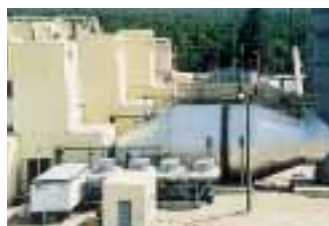
Gas turbine stations 'Millbank' and 'St. Rosé' in New Brunswick, Canada. Ten multi-layer expansion joints with diameters of 7.2 m and 4.2 m respectively, are installed after the turbine (ABB 11N) and in the duct leading to the chimney.
