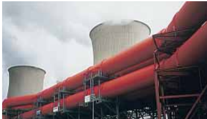
The FGD 'RWE' power plant Niederaussem, Germany.
