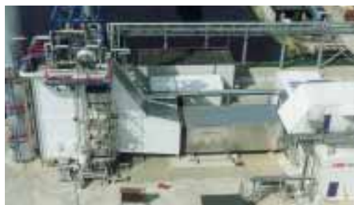
▲ Co-generation plant 'Hunze-Ström', the Netherlands. Generates energy and process heat for the production of potato starch. Gas turbine plant (ABB GT10) equipped with KE-Burgmann Combine-X® expansion joints.
