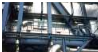
Combined cycle power plants 'Paka' & 'Pasir Gudang', Malaysia with Siemens V94.2 gas turbines. Combine-X® and Fluaflex® expansion joints are installed after the gas turbine and on the boiler. Medium: flue gas; t: ...590 °C (1,094 °F); p: -50...+70 mbar; Axial compression: ... 170 mm; Lateral offset: ... 125 mm
